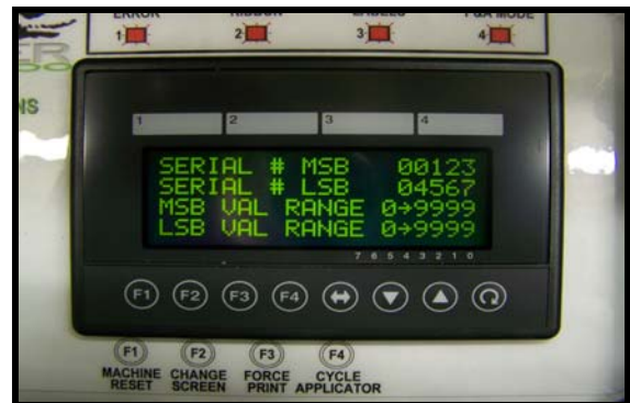
Figure 2: Panther 2000 display for setting the start value and displaying the current value
